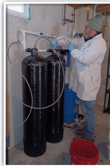
Collecting a sample from a point-of-entry water filtration system
